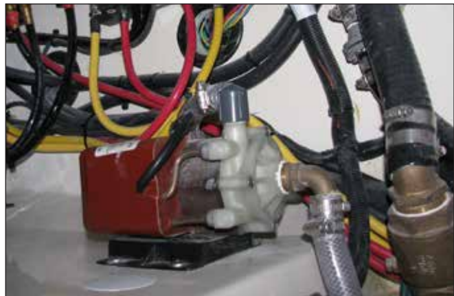
Air Conditioner Seawater Cooling Pump
