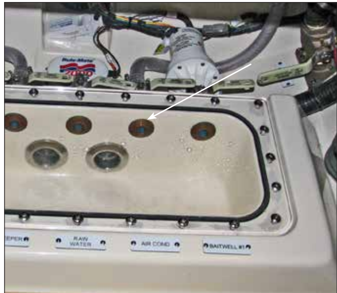
Air Conditioner Cooling Pump Supply Valve Fitting
