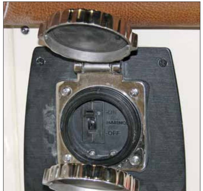
Shore Power Inlet Circuit Breaker
