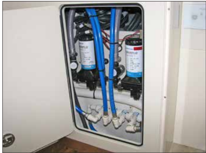
Fresh Water Pump Access Panel In Shower
