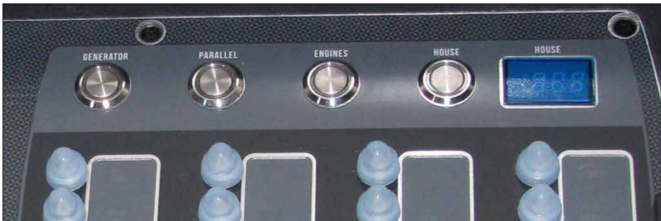
Cabin DC Panel Remote Battery Switches
