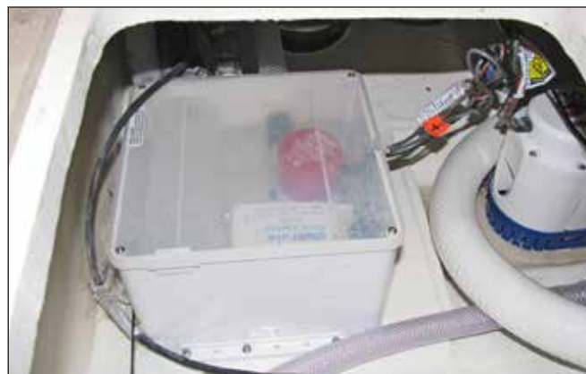
Shower Sump System In Head Compartment Bilge
