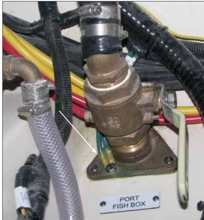
Thru-Hull Valve Bonding Wires & Connection
