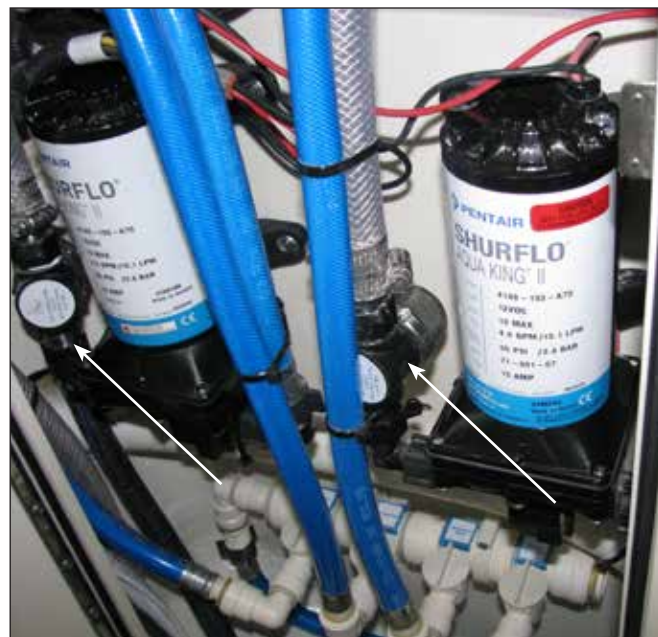
Fresh Water Pump Strainers
