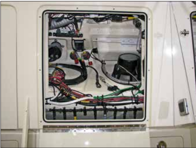
Helm Access Panel Above Marine Toilet
