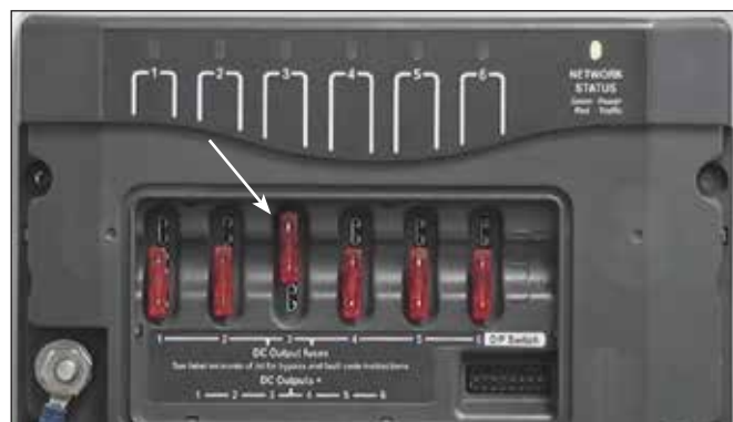
CZone Circuit 3 Fuse In Bypass Position
