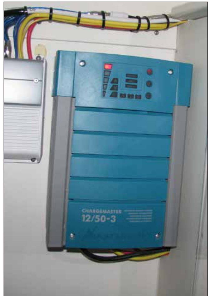
Typical Battery Charger
