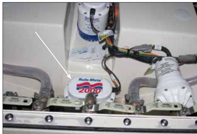
Aft Bilge Pump With Automatic Switch
