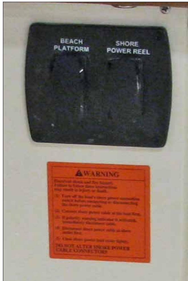
Shore Power Reel Switch
