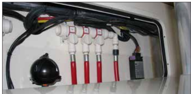
Hot Water Shutoff Valves Near Water Tank
