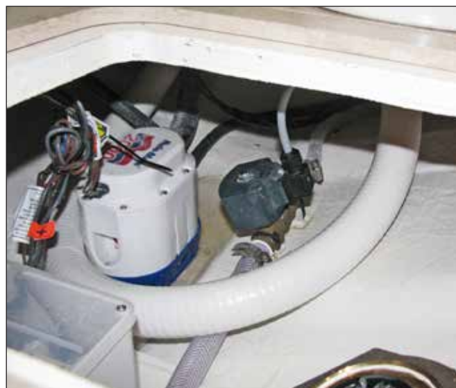
Forward Bilge Pump With Automatic Switch
