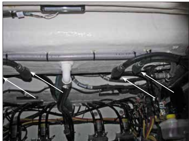
Fuel Primer Bulbs In Aft Systems Room
