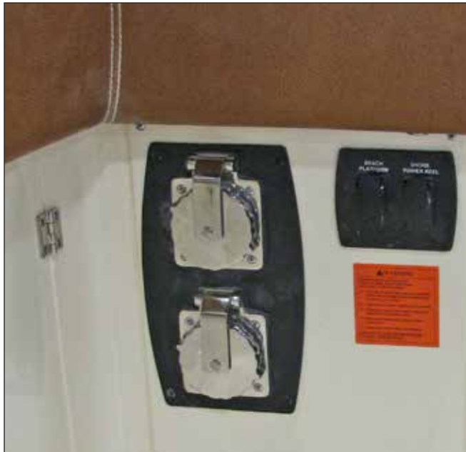
Shore Power Inlet Breaker & ELCI Inlet Panels
