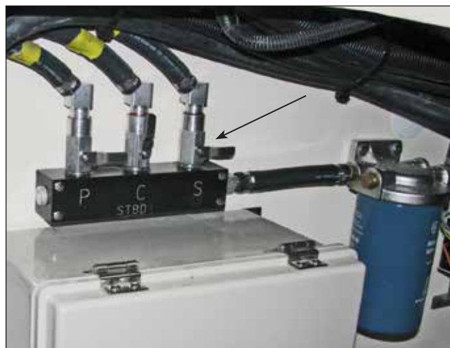
Stbd Engine Fuel Manifold & Valves
