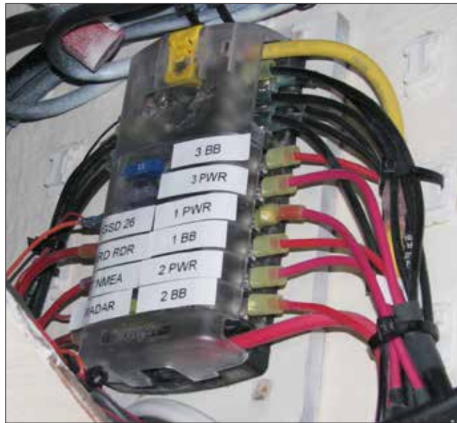
Electronics Fuse Panel
