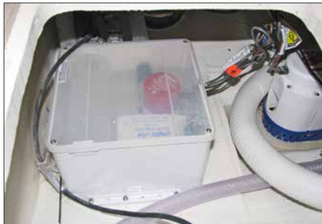
Sump Pump System In Forward Bilge
