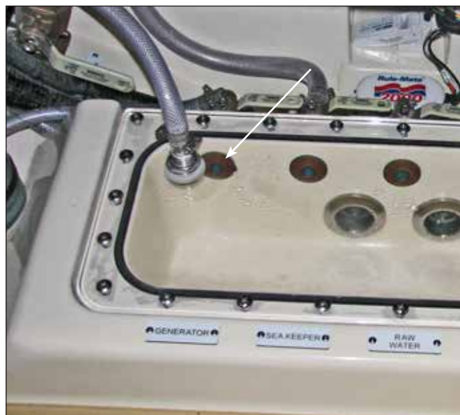
Generator Cooling Pump Supply Valve Fitting
