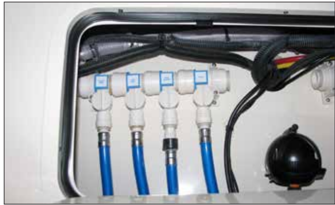
Cold Water Shutoff Valves Near Water Tank
