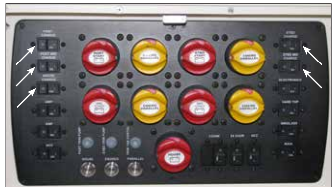
Battery/Charger Circuit Breakers
