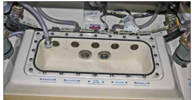
Generator Seawater Supply In Sea Chest
