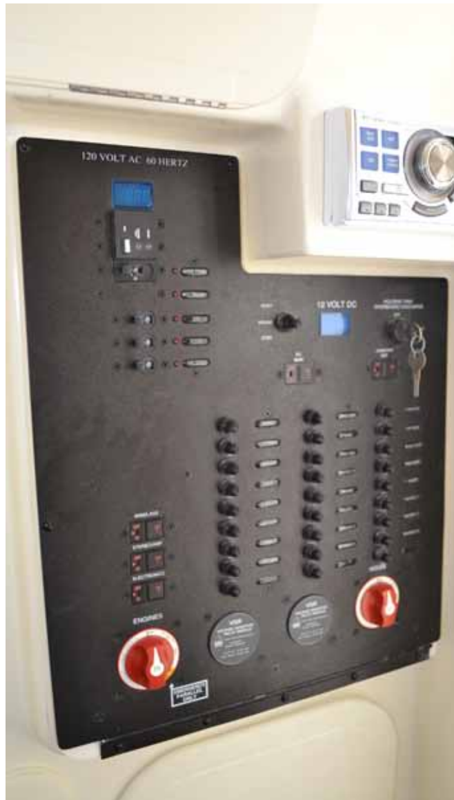
Battery Switches (red)
